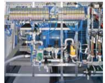
Clear installation of the control system for the VG
